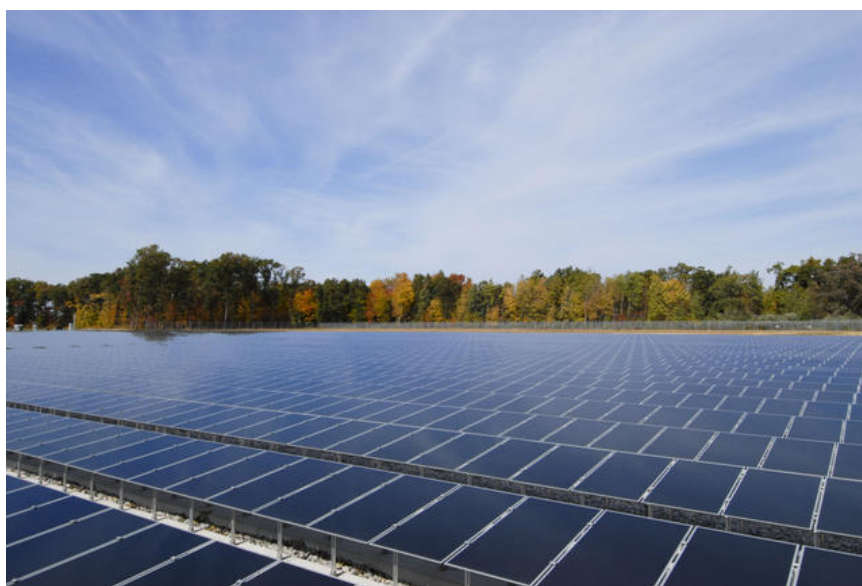
A solar field belonging to the 180th Fighter Wing, Ohio, Air National Guard, a project funded by DOD’s Defense Research and Development Program. Once completed, this field will allow the fighter wing to save approximately 37.5% on its annual electric bill. Courtesy of U.S. Air Force, photo by Master Sgt. Beth Holliker.
