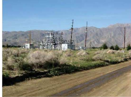
Figure A2: SDG&E's Borrego Springs Substation
