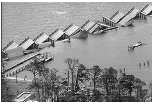
FIGURE 2 Damage from Hurricane Katrina to the Bay St. Louis Bridge in Mississippi. Source: NASA Remote Sensing Tutorial.
