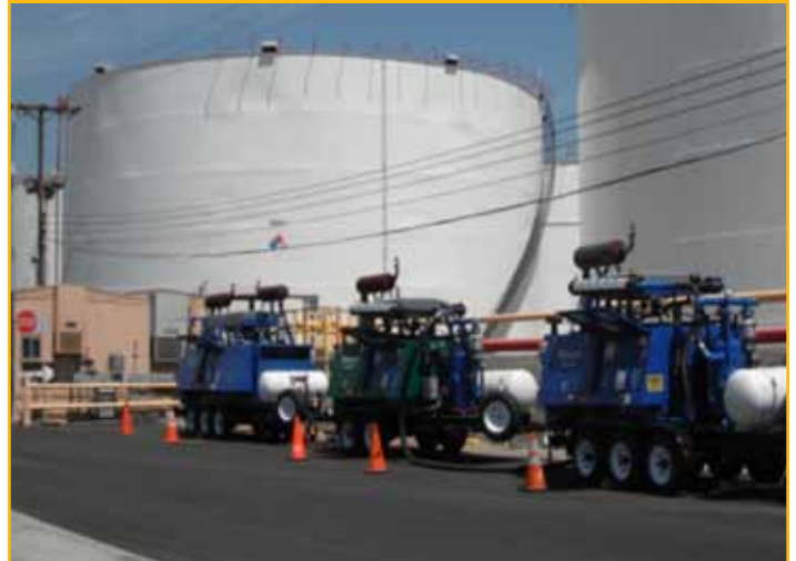
Figure 31: Vapor Recovery Unit
