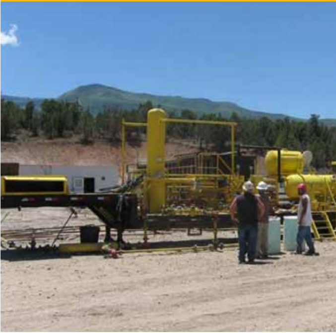
Figure 12: Green Completion Equipment
