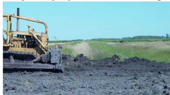
A bulldozer fills a drainage ditch as part of a wetland restoration on the Glacial Ridge property (TNC).
