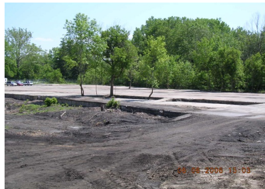
South end of the mill site after the demolition was completed (NPS).
