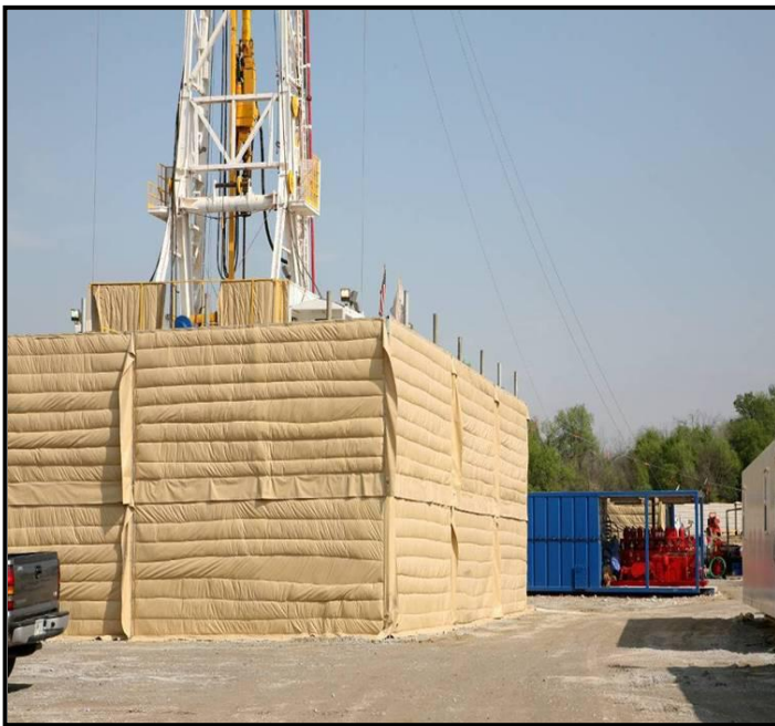
Source : Chesapeake Energy Corporation, 2008 Insulation Blankets Used to Deaden Noise from Drilling Operations
