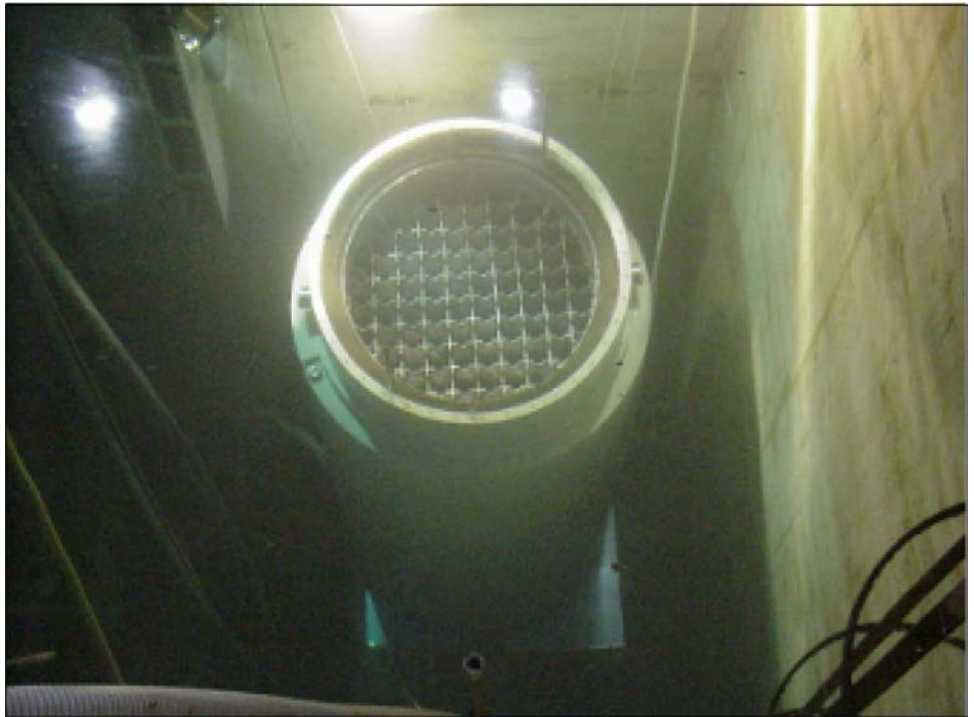
Figure 5: Canister in a Transfer Cask in a Spent Nuclear Fuel Pool
