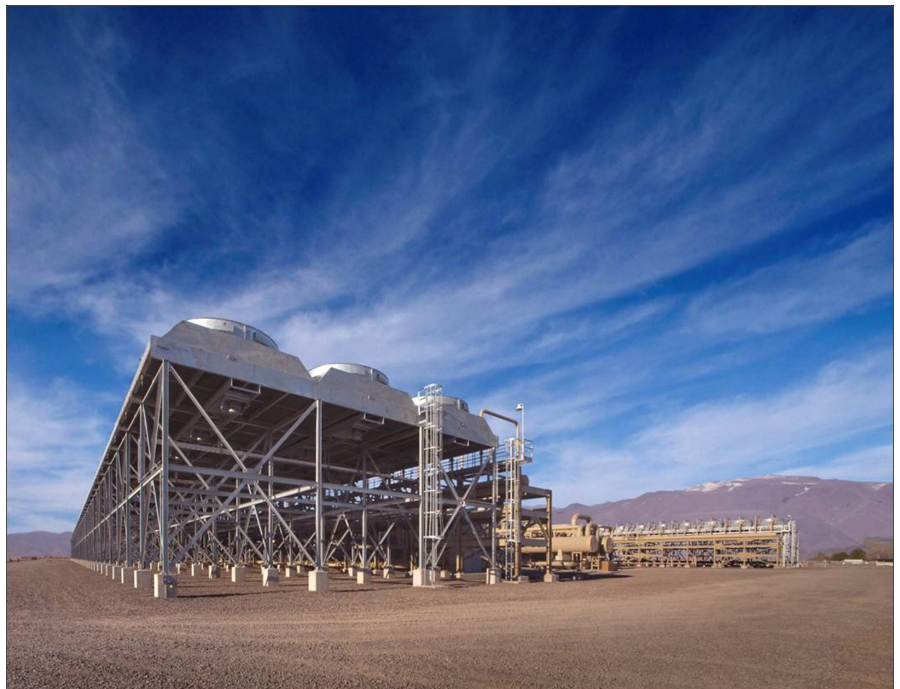
Enel's Stillwater geothermal power plant, Churchill County, Nevada. Photo courtesy Enel North America.
