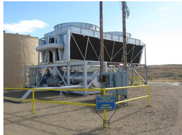
Figure 7: Binary plant recovering heat from coproduced oilfield water at Rocky Mountain Oilfield Testing Center RMOTC in Wyoming, Johnson and Walker (2010).
