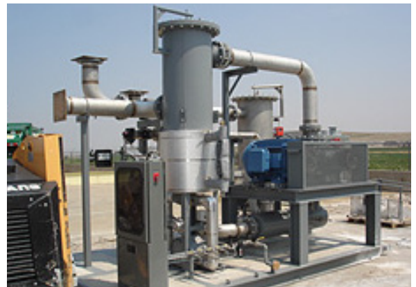
The plant at Lowry Landfill and an adjacent site will generate 3.2 megawatts of power annually. Source: Waste Management
