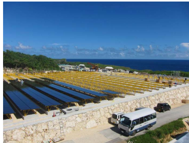
PV panels in Miyako-island
