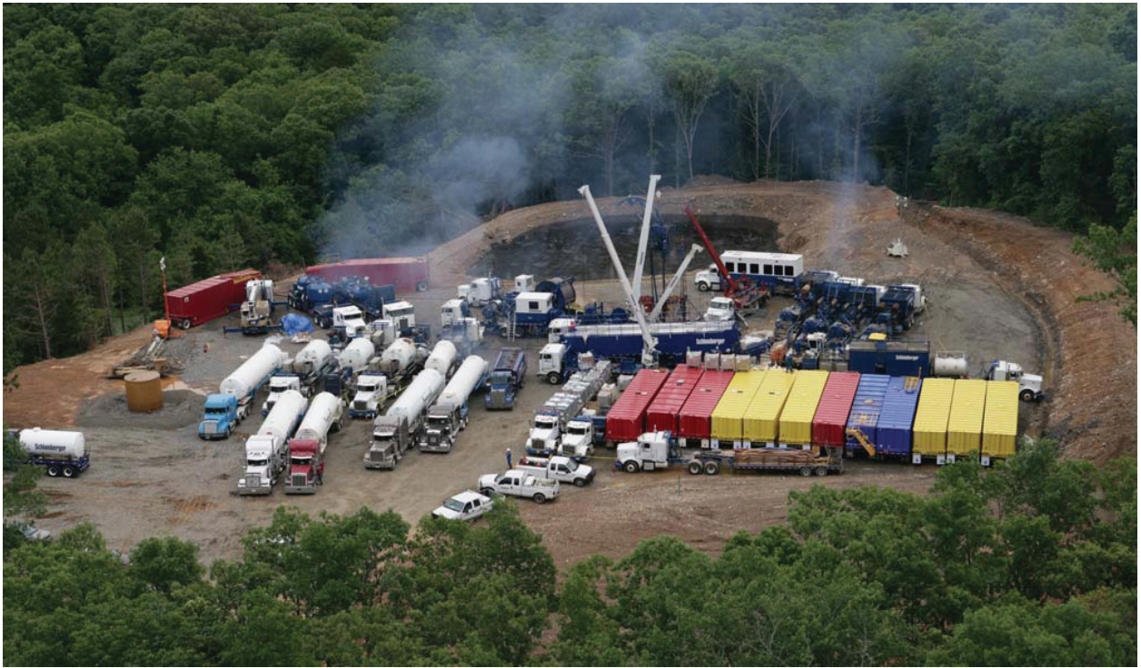
The numerous truck-mounted pumps and temporary storage tanks needed to fracture-treat the Marcellus Shale will require larger well locations. The fracturing equipment and materials on location in this photograph represent over 100 round trips to location by large tractor trailer trucks.
