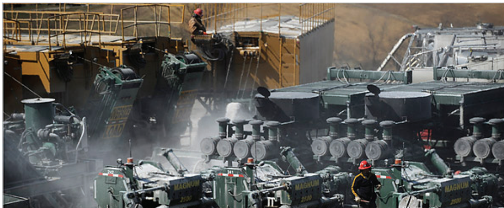
Typical equipment on a gas well site
