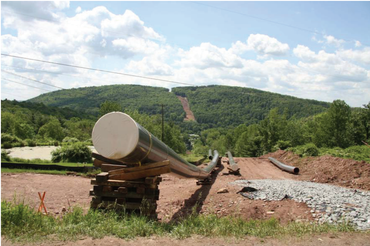
The Millennium Pipeline will allow for increased amounts of natural gas to be transported in New York State. Photo by David B. Soete.
