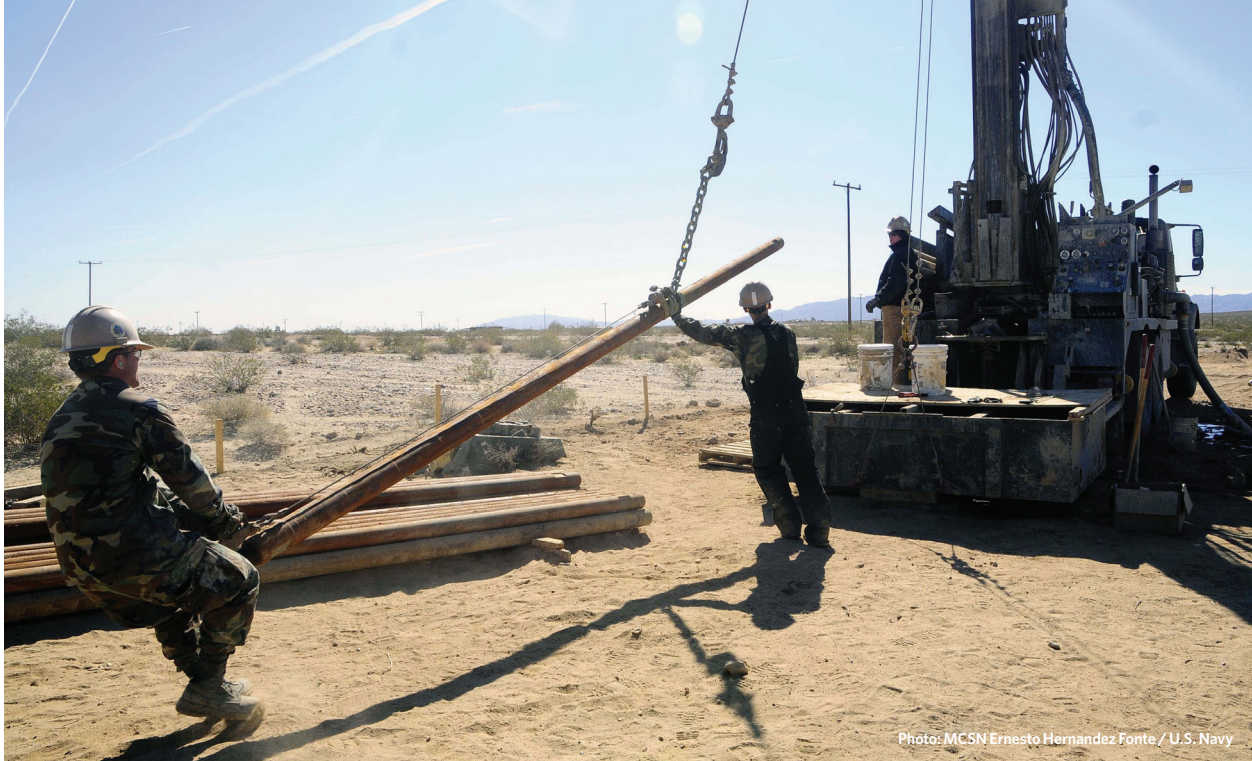
U.S. Navy Construction Electrician 3rd Class Robert Schiller, left, and Construction Electrician Constructionman Greg Langdon add a new section of drill steel to a T2W Ingersol-Rand Water Well-Drilling Rig in Twentynine Palms, CA, in 2009. Seabees from Naval Mobile Construction Battalion 1 drilled three 800- to 1,000-foot holes in the area to assist the U.S. Navy Geothermal Program Office in their research of local geothermal energy potential.
