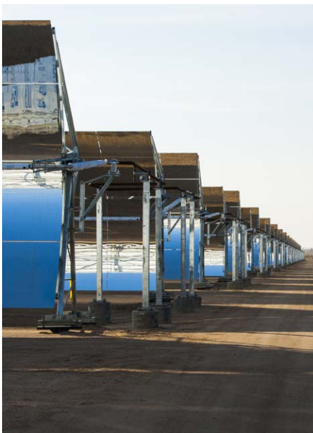
Mojave features DOE-supported parabolic trough technology to produce 250 megawatts of power. Photo Credit: Abengoa Solar, Inc.
