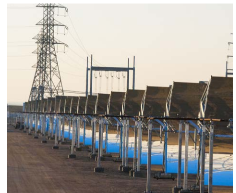
Mojave, Photo Credit: Abengoa Solar, Inc.
