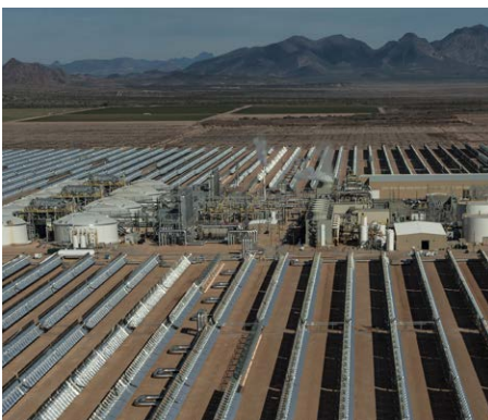
Solana, Photo Credit: Abengoa Solar, Inc.
