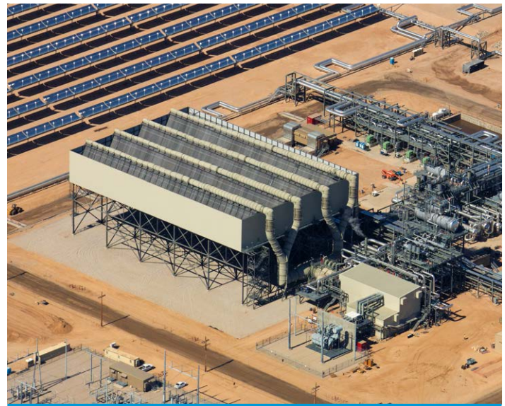
Genesis is expected to produce nearly 700 gigawatt-hours of renewable electricity each year from more than 500,000 parabolic mirrors.
