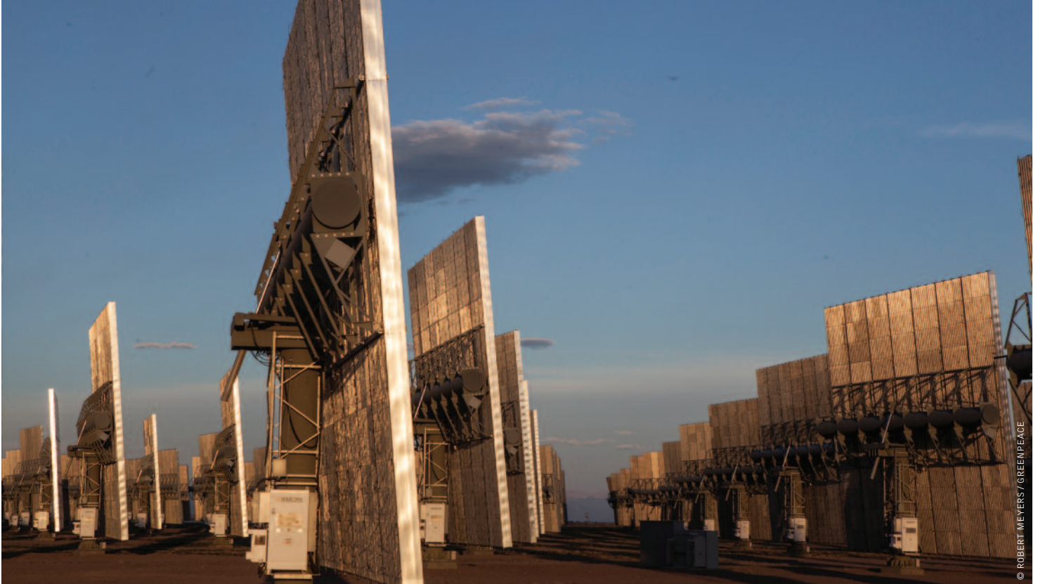
image ALAMOSA SOLAR GENERATING PLANT, COLORADO. A 30 MEGAWATT CONCENTRATING PHOTOVOLTAIC (CPV) POWER PLANT OWNED BY COGENTRIX ENERGY. IT WAS CALLED THE LARGEST CPV FACILITY IN THE WORLD WHEN IT CAME OPERATIONAL IN MAY 2012
