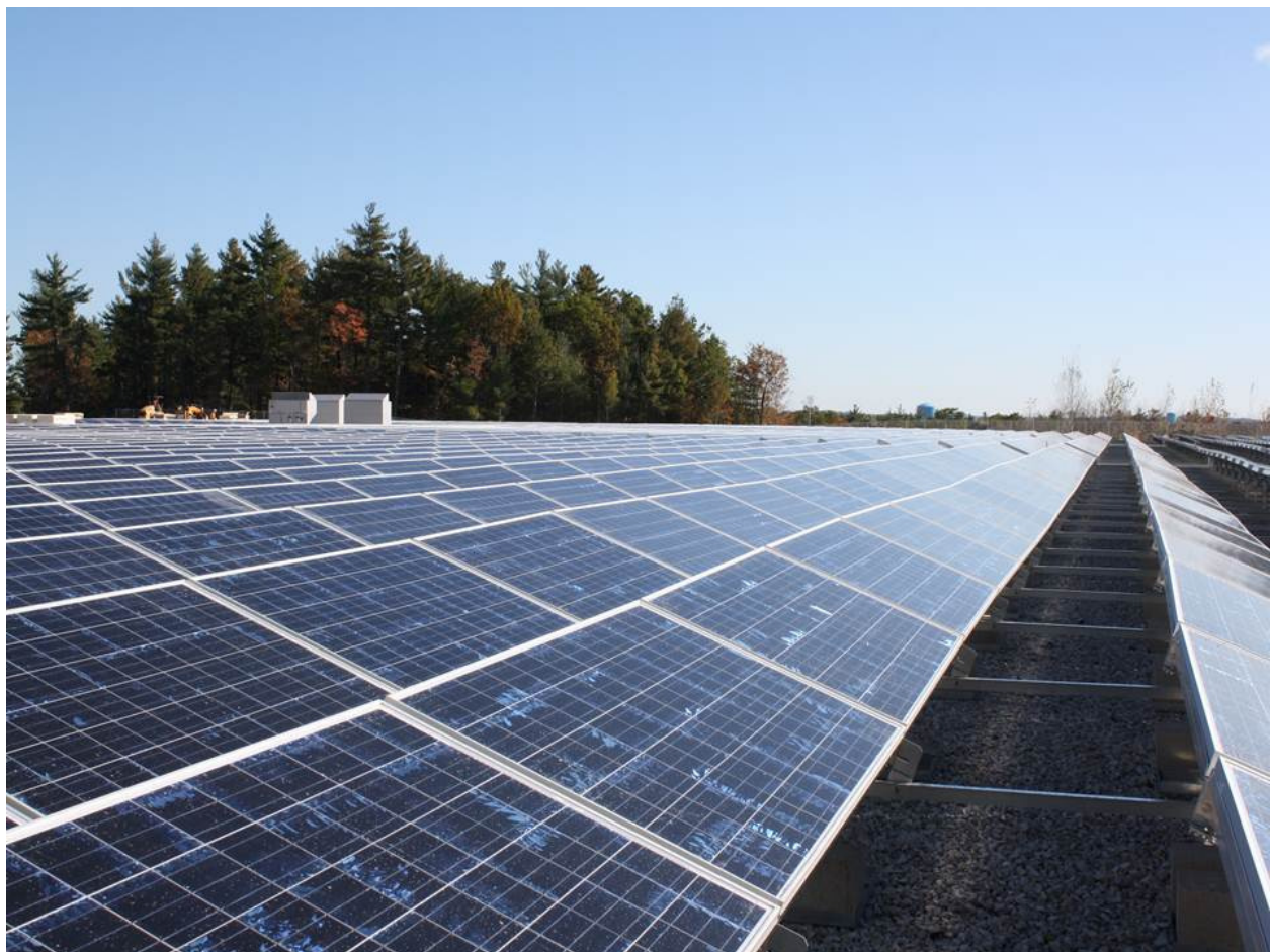
Westford Solar Park, photo courtesy of EEA
