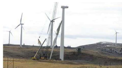
Wolverine Creek Wind Turbines in Idaho
