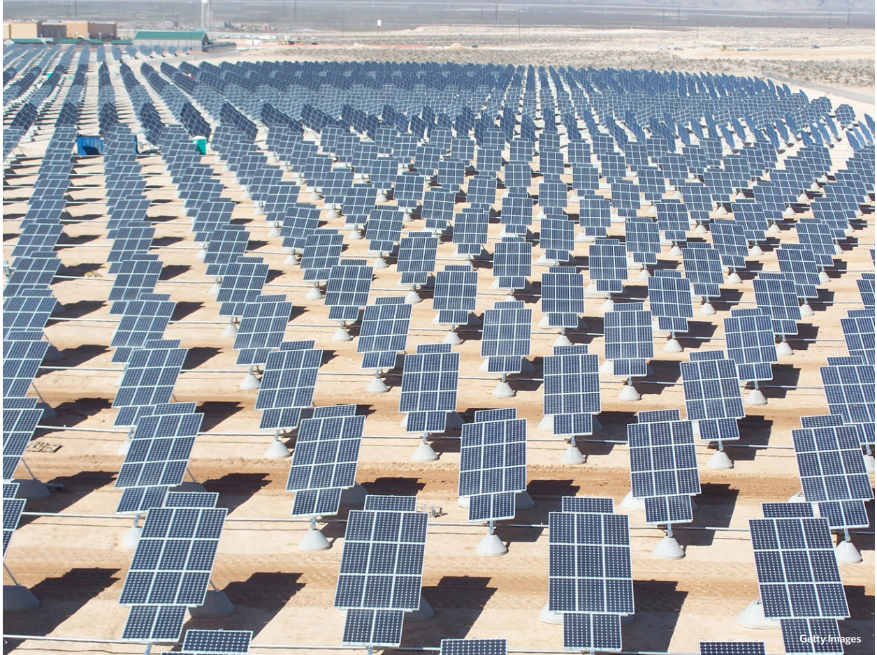
Solar installation at Nellis Air Force Base in southern Nevada.
