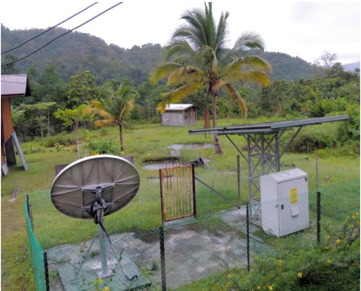
Figure 2: A village micro-grid energy and telecommunications system in the Crocker Highlands of Sabah, Malaysian Borneo. The system serves a community of two hundred, and provides household energy services, telecoms and satellite (dish shown), water pumping for fish ponds (seen at center) and for refrigeration. The supply includes micro-hydro and solar generation (one small panel shown here, others are distributed on building rooftops). Photo: DM Kammen.
