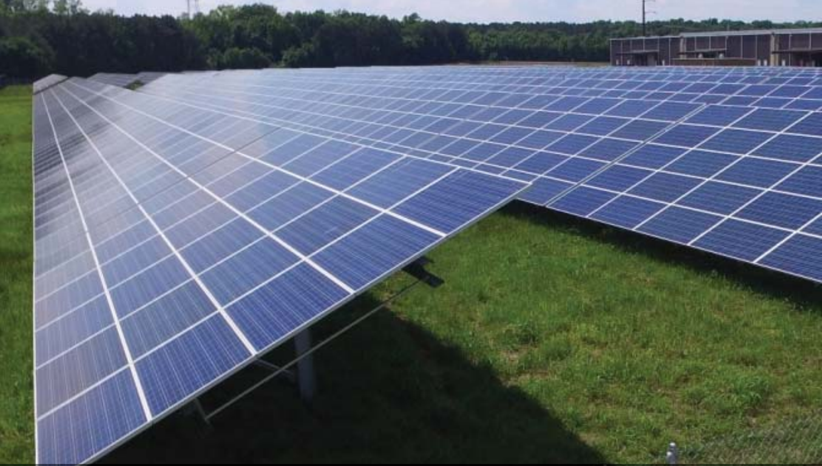
2000 KW AC ground mounted solar array installed at Philip Morris' Park 500 facility on Bermuda Hundred Road PHOTO CREDIT: DOMINION VIRGINIA POWER
