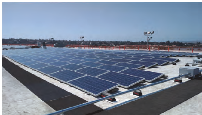
Figure 7-4. Solar photovoltaic on the roof of Terminal 2 at San Diego Airport.
