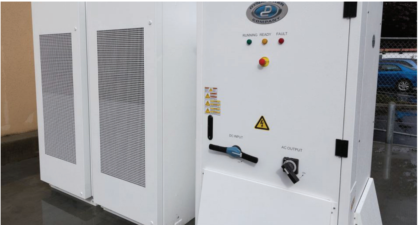
Installation: Sprigg Electric — 250KW MPS-250 coupled with Tesla batteries San Jose, CA
