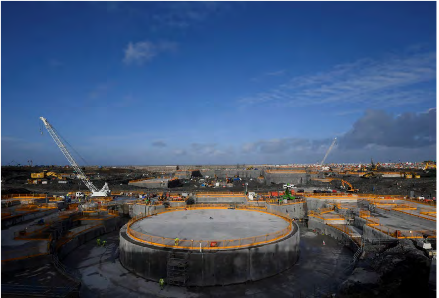
Construction including one of two 'nuclear islands' is seen at the Hinkley Point C nuclear power station near Cannington in southwest England, January 17, 2018. Source: REUTERS/Toby Melville.
