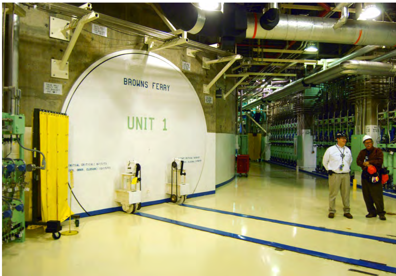
Nuclear officials stand near the entrance to a reactor at the Browns Ferry nuclear facility in Alabama, in this photo taken March 25, 2011. The Browns Ferry nuclear plant, similar in design to the earthquake-hit Fukushima facility in Japan, has multiple defenses installed after 2011 to prevent and tackle the same kind of emergency, its operator said. Picture taken March 25, 2011. Source: REUTERS/Matthew Bigg.
