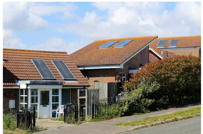
Fig. 4. Discoloured and corroded solar panel systems in need of cleaning or repair in Whitehawk.
